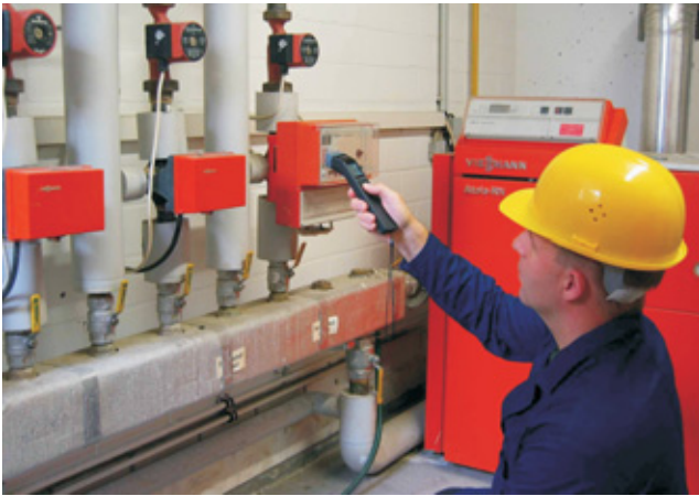
Checking the temperature of heating circles
